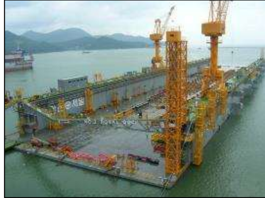
The world's largest floating dry dock will soon be Royal Dock 5, 432 by 86 meters. Above, Royal Dock 3, as 5 is in construction. 16 pumps can raise or lower the dock by 21 meters in 3 hours.
